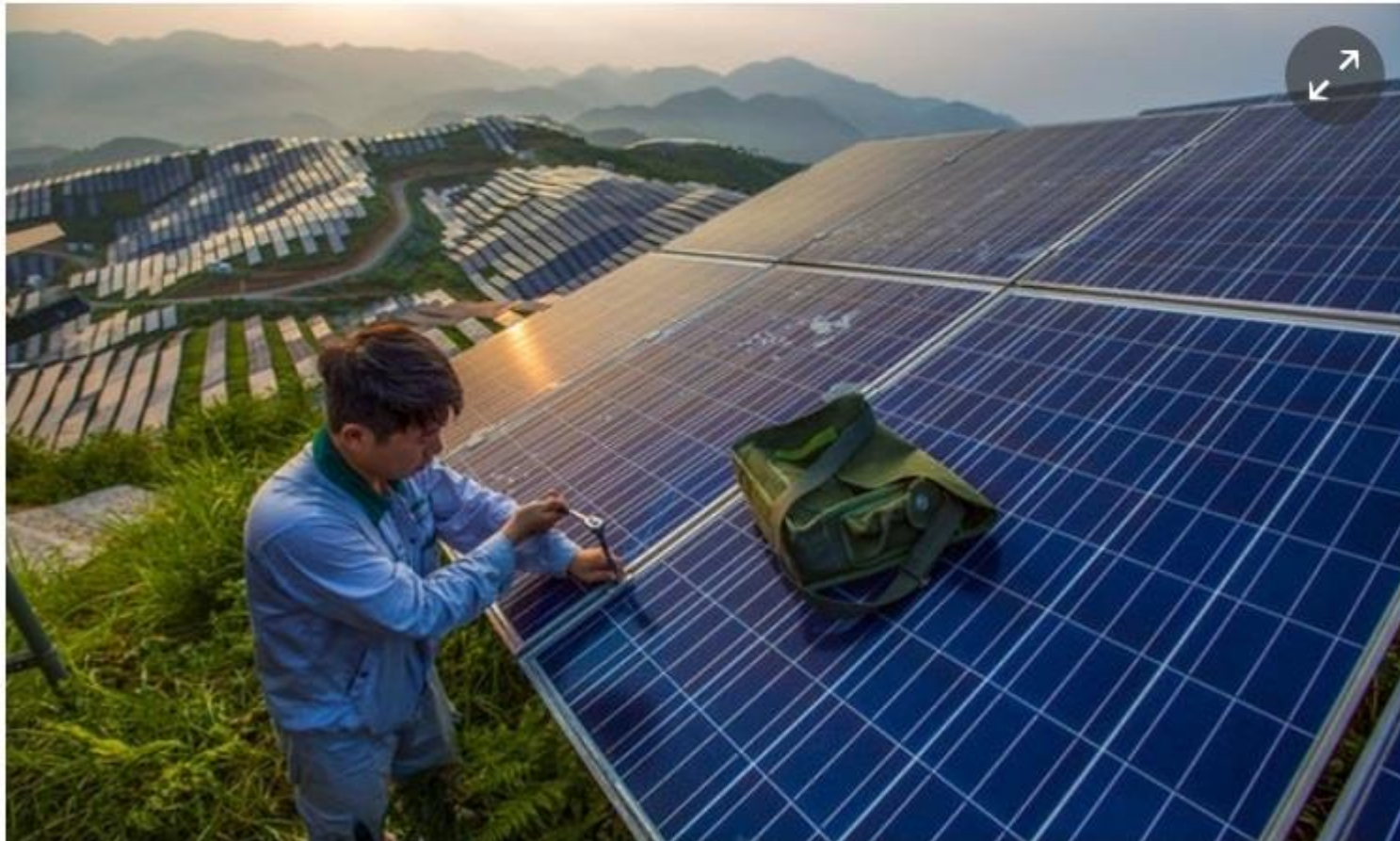
i A worker maintains photo-voltaic panels at Xinyi station in Songxi, China. Photograph: Feature China/Barcroft Images
